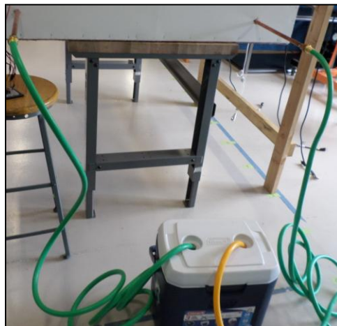
Figure 4.20: The Outside Components of the A/C System
